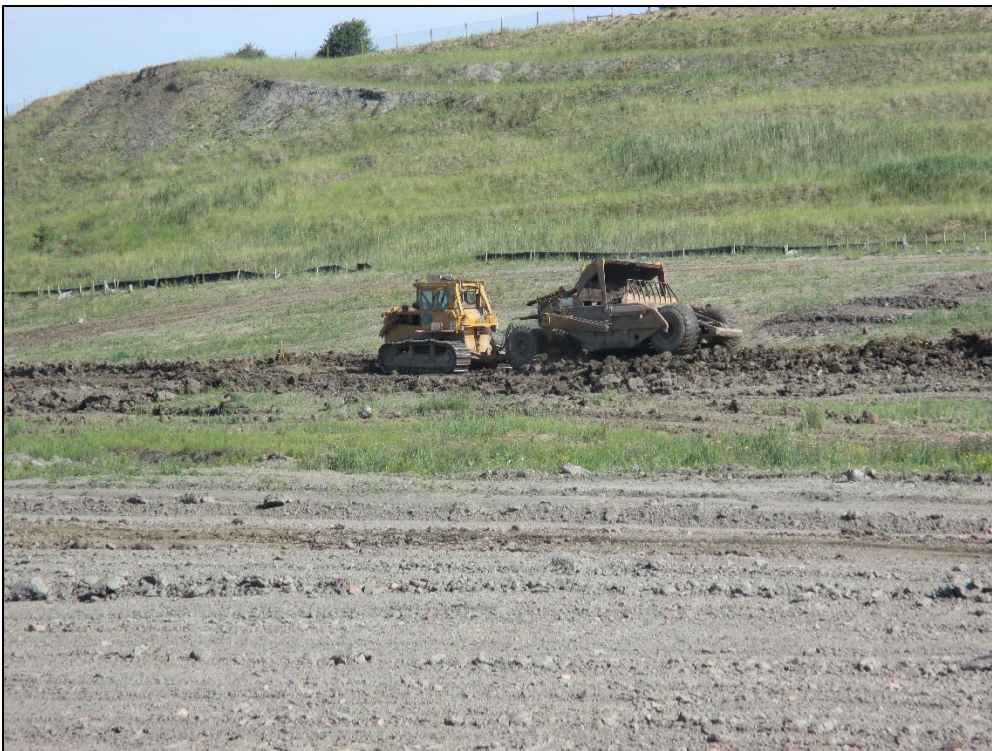
Photograph 2 – Facing broadly east at vegetated and terraced eastern slope face of Rookery South Pit.
